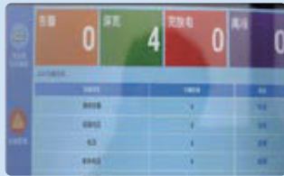
Data Centre Battery Status Monitor System
