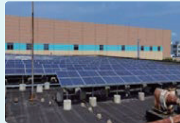
Photovoltaic power generation system
