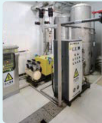
Device for reuse of reclaimed water
