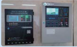
Data Centre Fire Fighting System
